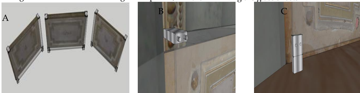
Figure 6 A The final view of the special glass on mural paintings, (B ,C) The shape of the nails which used in the installation of the glass to the wall
